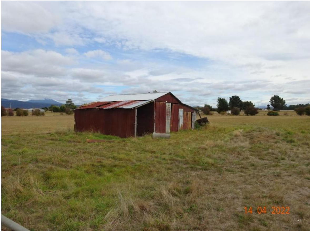
Figure 4: Dilapidated agricultural building.
