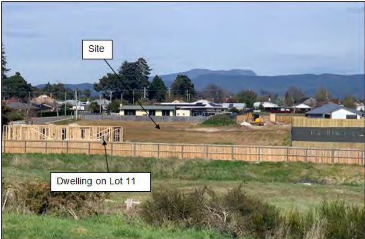
Photo 2: At the railway line looking south towards the site. The dwelling being constructed is on Lot 11 of Planning Permit PA\19\0053.
