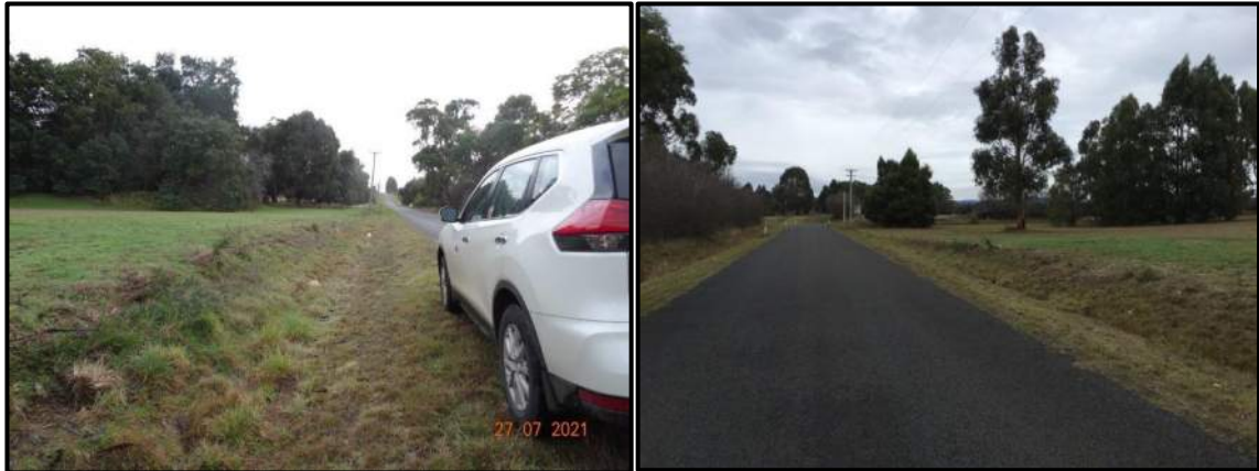
Photo 9 & 10: Looking north and south along Five Acre Row showing the open stormwater drain that is located in the road reserve.
