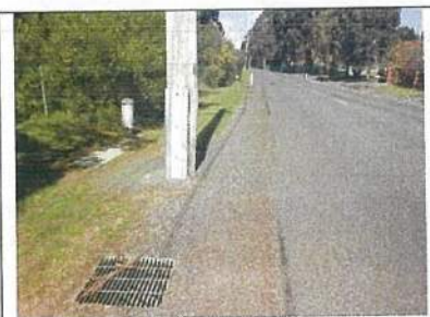
Figure 6 - Pole and pit
