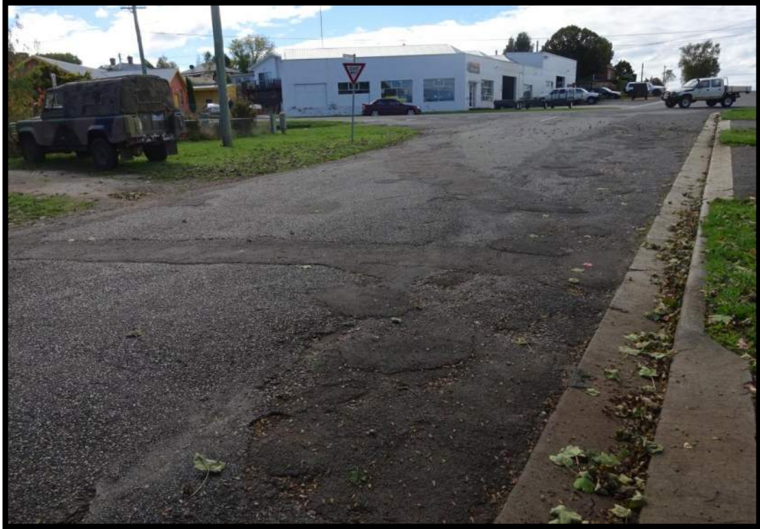
Photo 6: Beefeater Street to the north of the subject title, showing the existing road condition.
