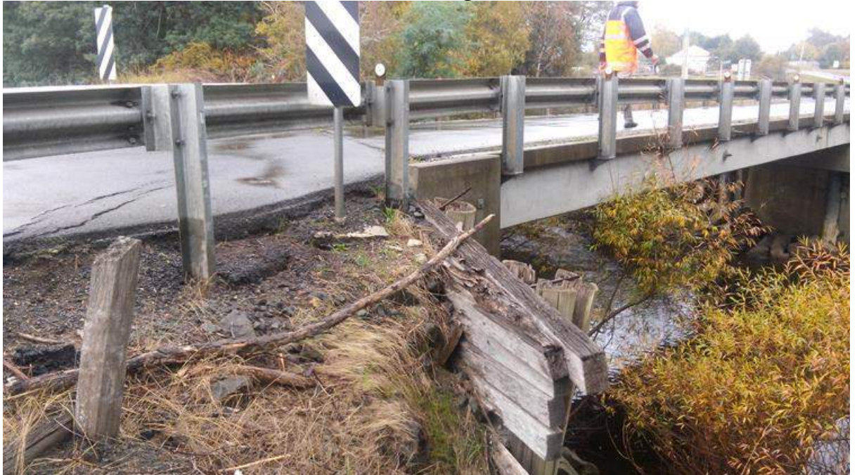
Photo 3: Eastern downstream abutment wingwall showing pavement stress
