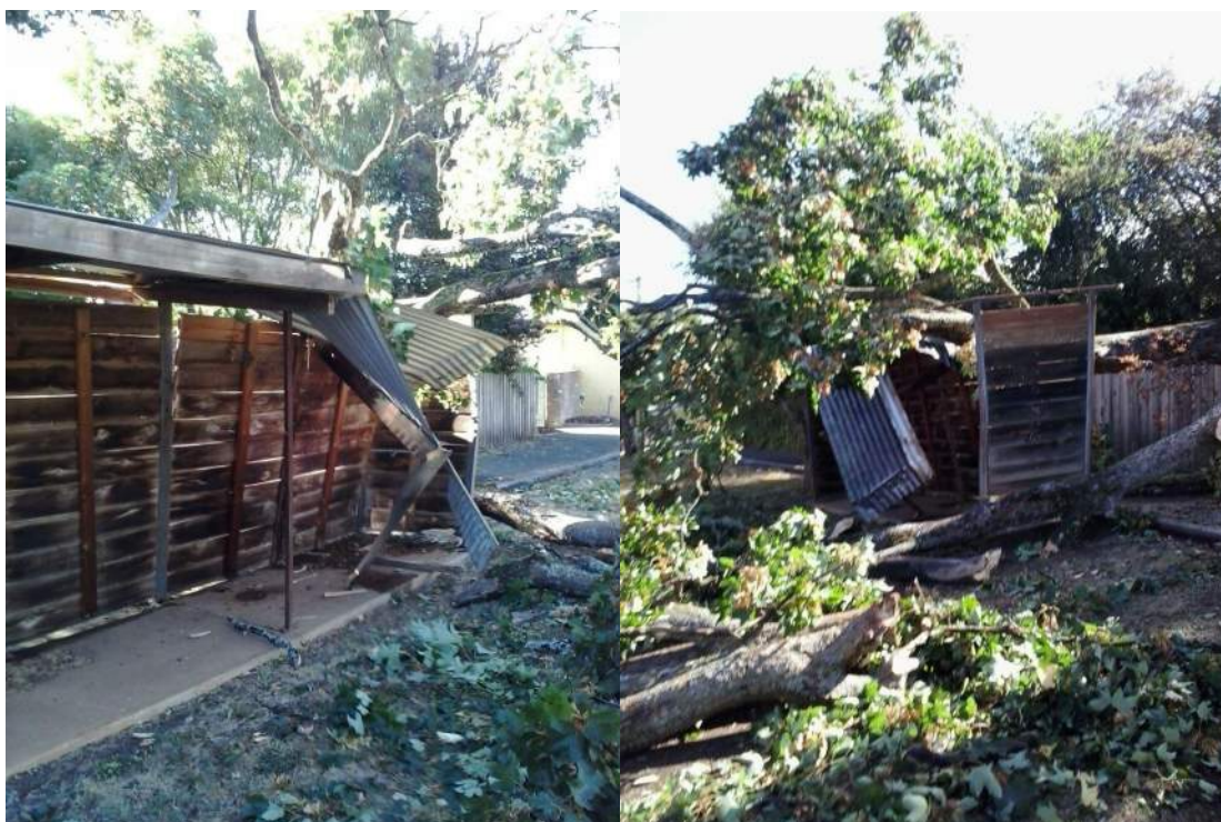
Photo 1 and 2 : Damage to existing timber bus shelter
