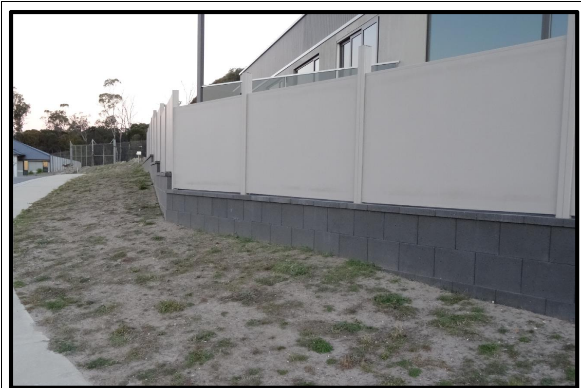
Photo 6: Existing fence at 5 Classic Drive, showing separation and impacts on the footpath.
