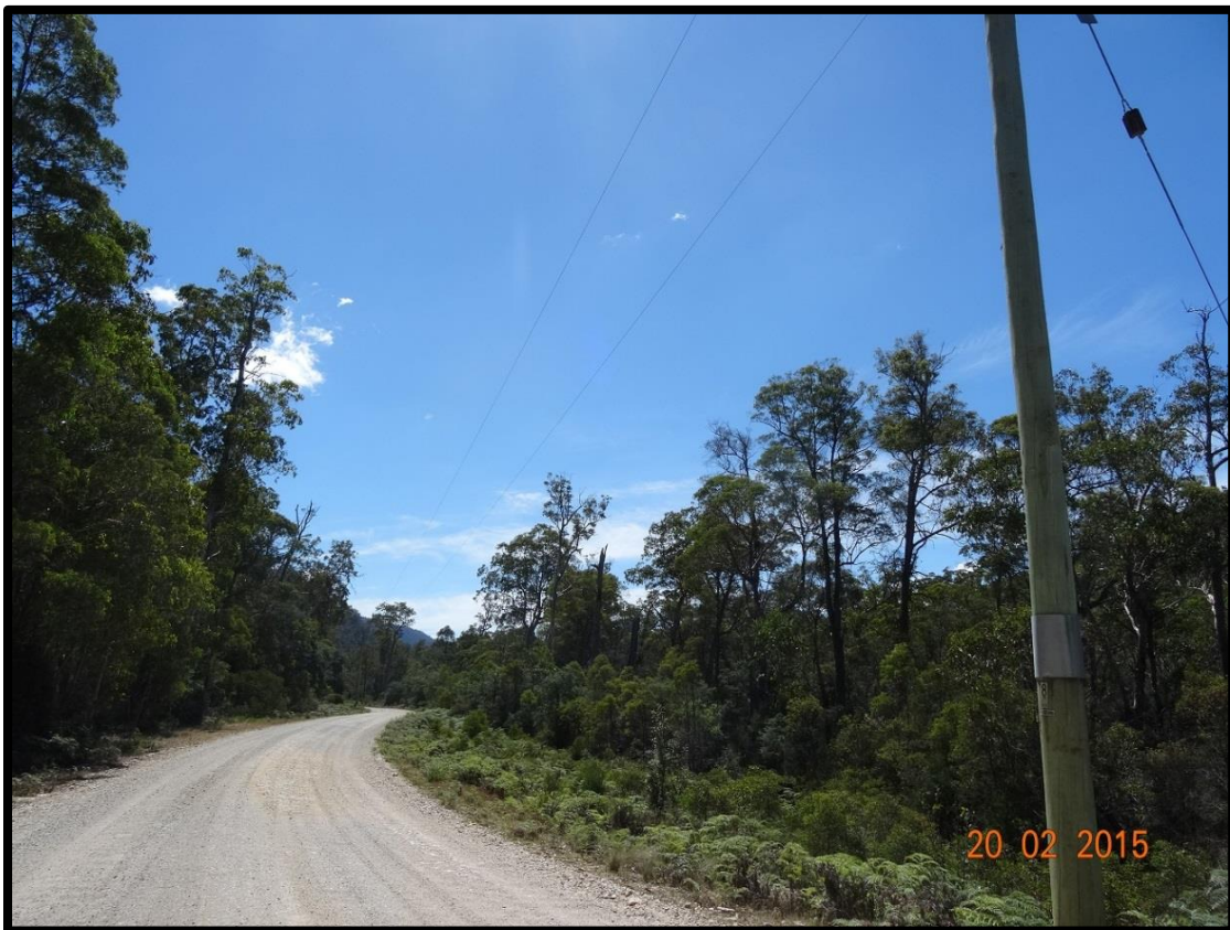
Photo 6: Mersey Forest Road to the north of Lake Rowallan, showing existing transmission lines.
