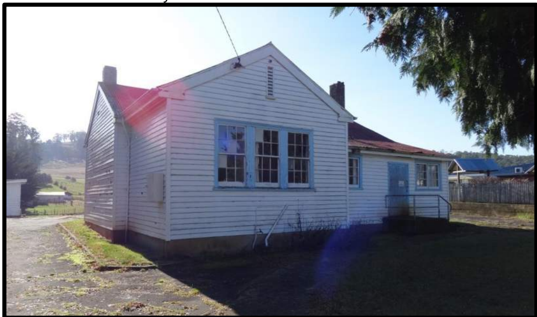
Photo 1: Subject school building proposed to be demolished, looking north from Pioneer Drive.
